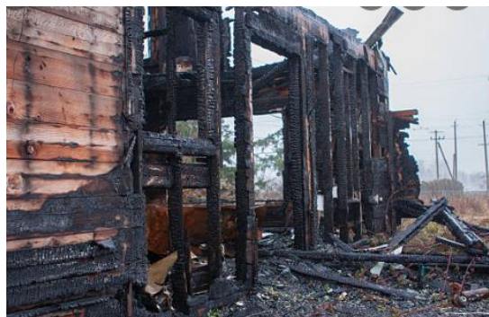
Figure 7. Wood fire damage
