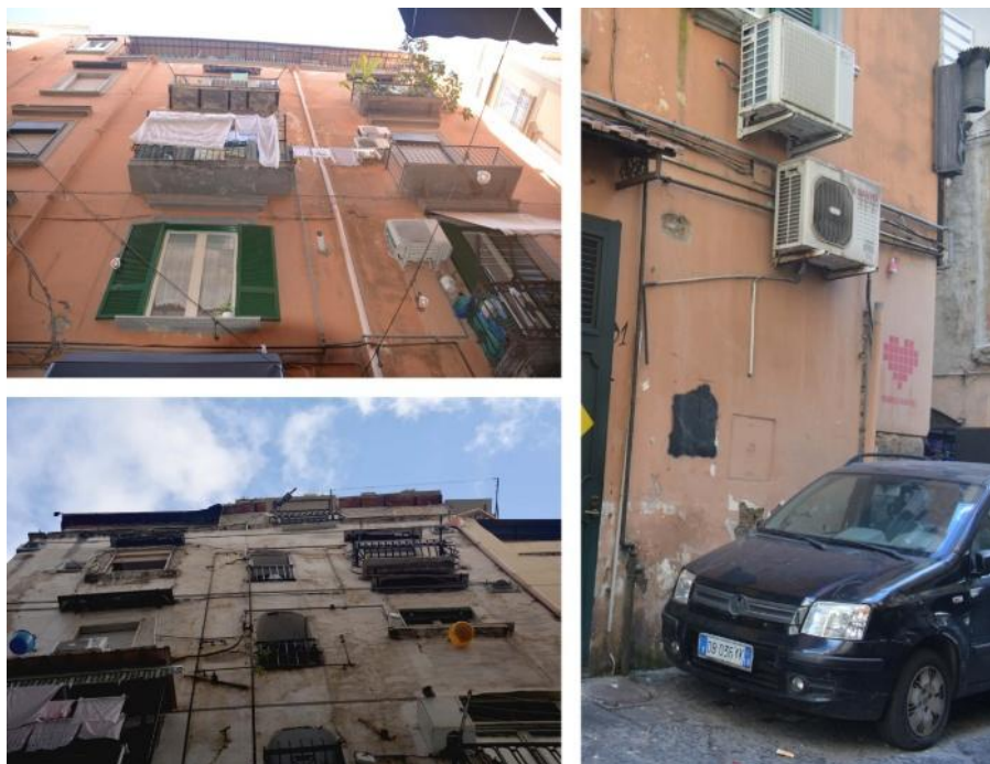
Figure 10. Poorly integrated installations within the compositional design of the façade
